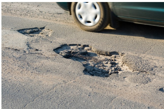
Figure 1: Potholes in Asphalt Roadway
